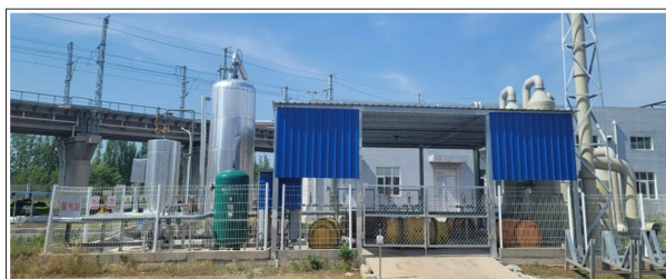
Figure 6: Ammonia Station for supply to test-cell
