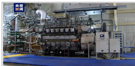
Figure 5: R&D test cell for the new ammonia dual-fuel engine 12V240H-DFA
